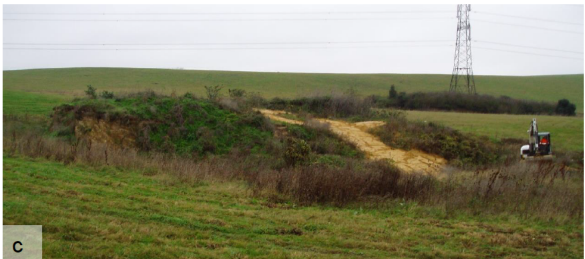
Figure 3. Baker's Hole Site B, in its setting: (a) general view of Sites/Areas B, C and F before devegetation of Site B in September 2014 [23-Feb-2012, looking SE]; (b) after devegetation [15-Sep-2014, looking S]; (c) after remedial backfilling in December 2015, with Area C in background [18-Jan-2016, looking NW]
